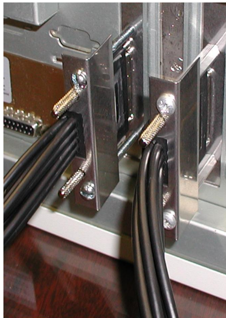
Figure 2-1: Installed Cards with Stability Bracket Accessories
